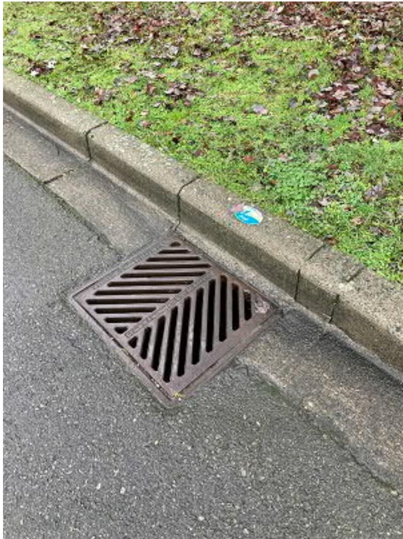
Picture 11: north side of intersection: SE 24 th Street and 63 rd Avenue SE This is a Type 2 catch basin, very big inside. From here water turns to the northwest and heads into Aubrey Davis Park.
