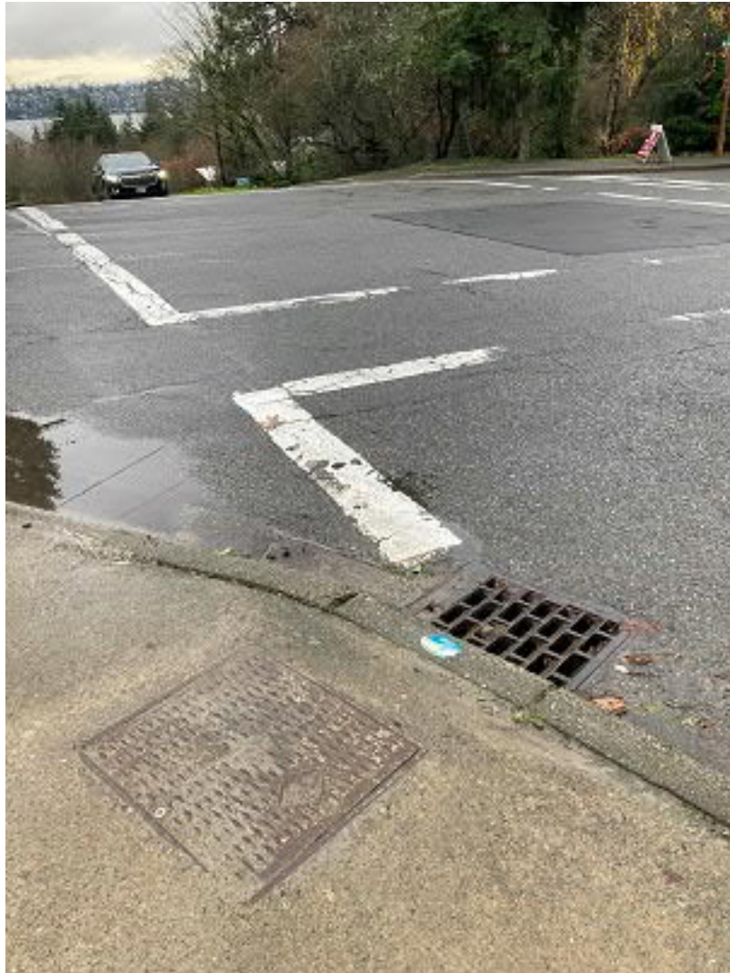
Picture 8: ROW at SE corner of SE 24 th Street and W. Mercer Way From here (solid lid), water crosses diagonally across the intersection.
