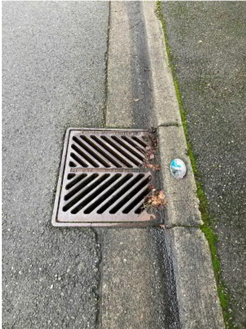
Picture 9: just west of NW corner of SE 24 th Street and W. Mercer Way Heading west under north side of SE 24 th Street
