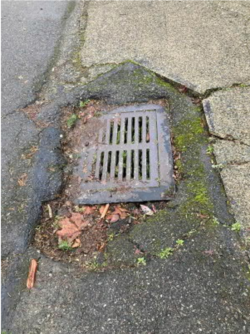
Picture 2: ROW between 2526 and 2520 70 th Avenue SE This is connection point for new house. Existing storm drain runs north under eastern ROW.
